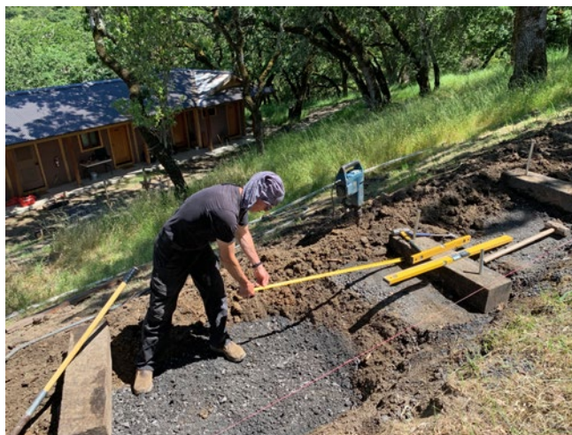
(Top) View of work in progress on pathway leading to the Genjo Building
